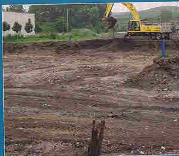
Russo excavated and removed PCB and VOC contaminated soils and installed a site-wide cap that consisted of a geotextile membrane, clean soil and various impervious surfaces such as pavement and building foundations.
