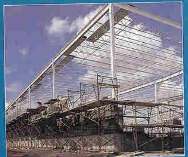
The Saw Mill Park project, seen here in July 2004, received up to 75 percent of its remediation costs because of the significant amount of state and local taxes anticipated from the project.
