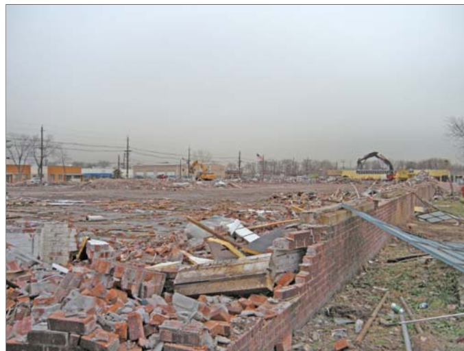
The demolition site of Kearny's mixed-use Schuyler Crossing, Russo Development's first such construction project. [Courtesy of Russo Development]
